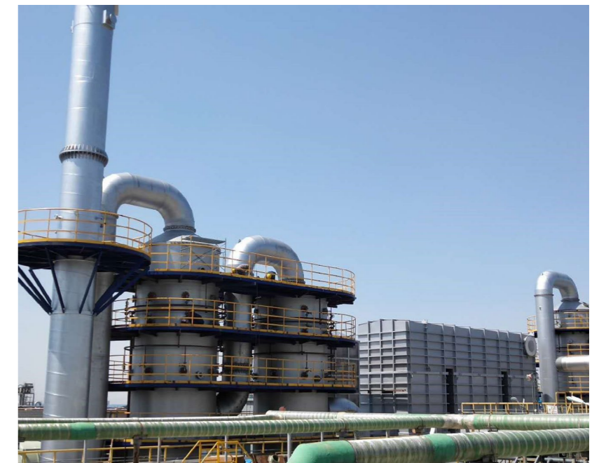
RTO exhaust gas incineration facility
